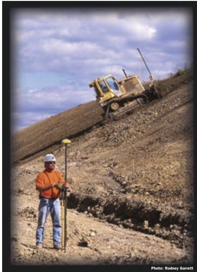
Some of the latest GPS technologies are being evaluated on this project.
