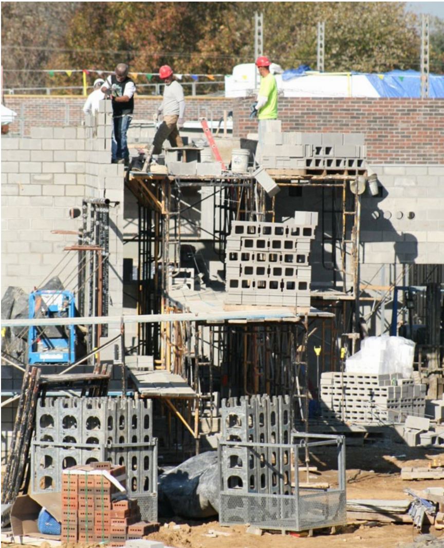
The increasingly important role of the National Guard, coupled with funds made available as part of the AARA of 2009, have increased new army construction in West Virginia.
